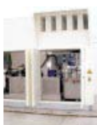
Station de compression GNV
