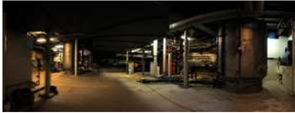
Installations techniques - piscine Guy-Berthier
